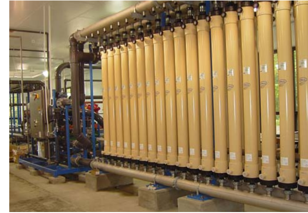
Membrane Filtration Unit
